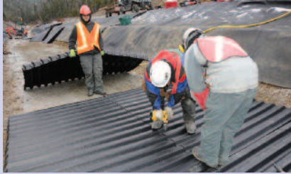
Weighing less than 75 lbs. each, the lightweight MegaDitch sections are easily moved into place.
