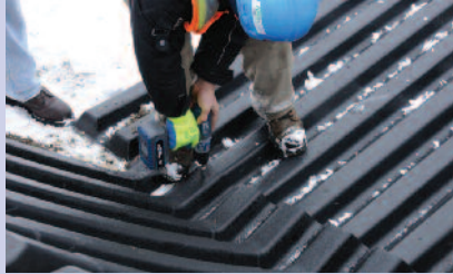
A handheld power drill is used to install the self-tapping, corrosion resistant screws that join each section.
