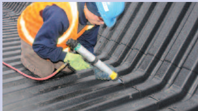
A water and weather resistant adhesive is applied to the seams between the base sections and the interlocking/overlapping sidewalls.
