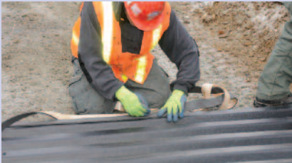
Gaskets are applied to each downstream section to seal the joints in the floor. The ribbed interlocking design ensures a snug fit.
