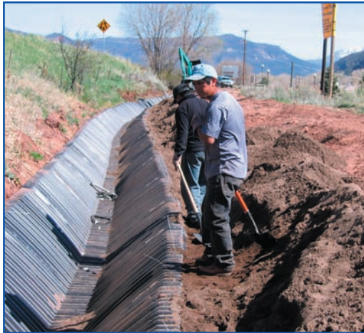
After installing and anchoring the SmartDitch sections, laborers backfill along the sides to match the existing grade.
