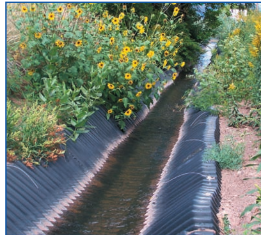
A couple of months after the installation, the natural vegetation has grown right up to the edges of the SmartDitch sections. The natural vegetation combined with the SmartDitch sections provide a stable waterway for the irrigation channel and a strong barrier against erosion on the hillside.
