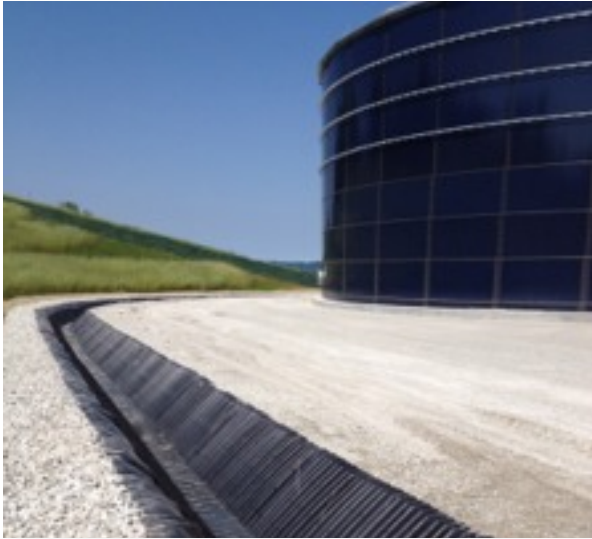
New water tanks were being threatened by slope-side stormwater run-off. SmartDitch solved the problem.
