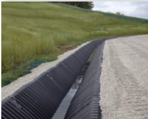
800' of 24" SmartDitch included several bends and curves to match the contour of this slope .
