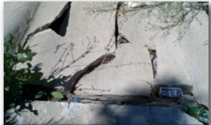
Failed non-reinforced concrete spillway.
