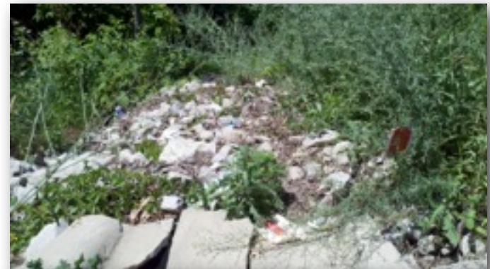
Rip rap repeatedly failed, and the drainage channel became overgrown.
