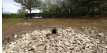
Pond's drainage inlet before SmartDitch
