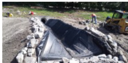
The SmartDitch flared-end section and edge protection further ensure improved drainage and minimal erosion will occur in the future.
