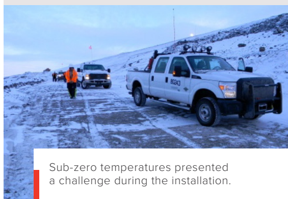
After a slow start to anchoring SmartDitch into the frozen ground, minor modifications were made to speed up the process.
