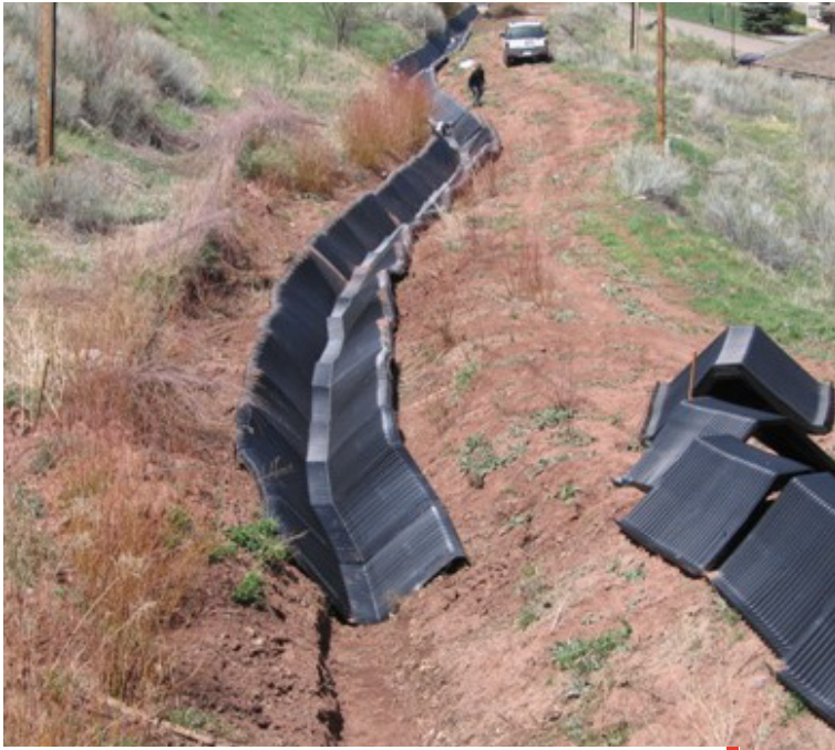
Site overview during construction. Photo shows the installation after the first day. The sections have been installed in the ditch with additional sections awaiting installation. This photo is prior to backfilling and final grading and shows the condition of the ditch after cleaning up the debris.
