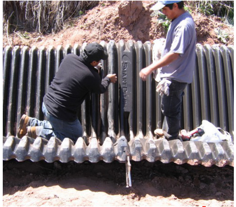
Site during installation of SmartDitch. Photo shows the quick and easy process of anchoring and installing SmartDitch sections.
